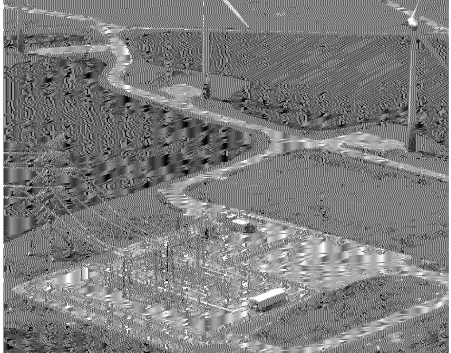
Existing Castle Rock Ridge Substation
